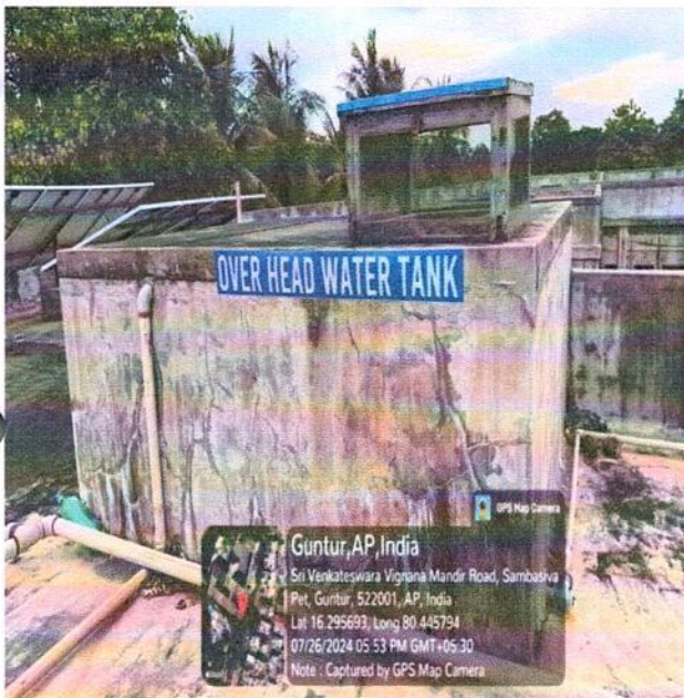
Hostel Block Water Tank
