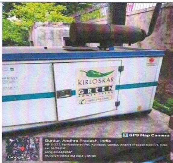
30 KV KIRLOSKAR Generator
