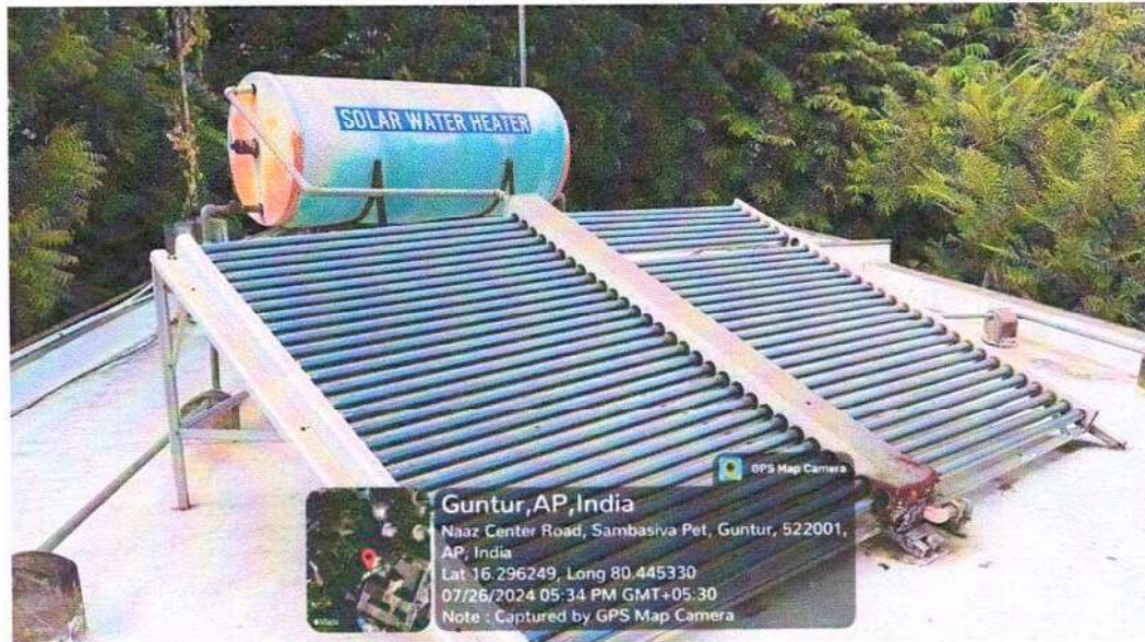
Solar water heater in Block - 1
